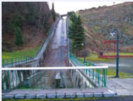
Present condition of slippage from flood banks on the dam reservoir Sance. Repair of slippage is the subject of the project “Reservoir Sance – transfer of extreme flooding”.
